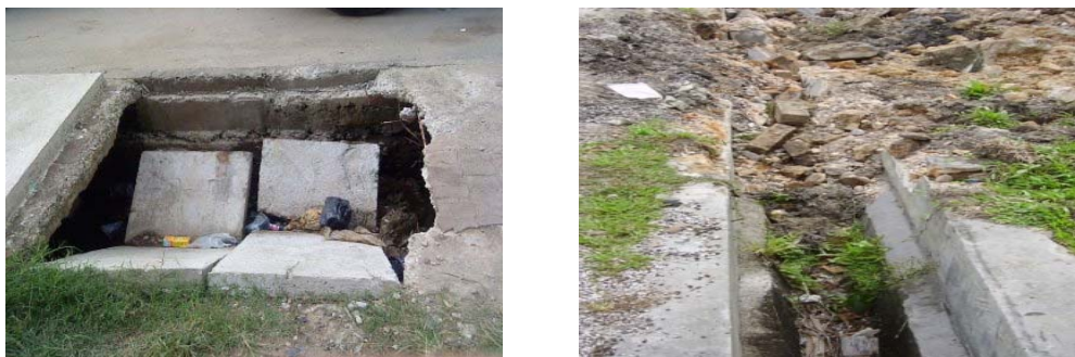
Figure AX2.7: Structure Failure
