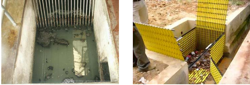
Figure AX2.5: Primary Outlets Clogging
