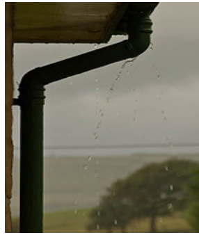
Figure AX2.3: Leaking Downpipe
