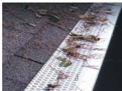
Figure AX2.2: Partially Clogged Gutter Screen
