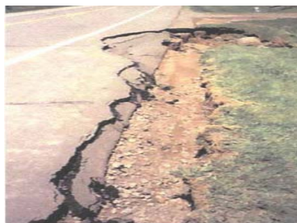
Figure AX2.8: Deterioration of Pavement Edge
